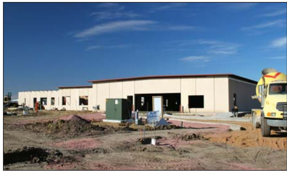
The Homeland Security facility under construction in Sioux Empire Development Park III.
