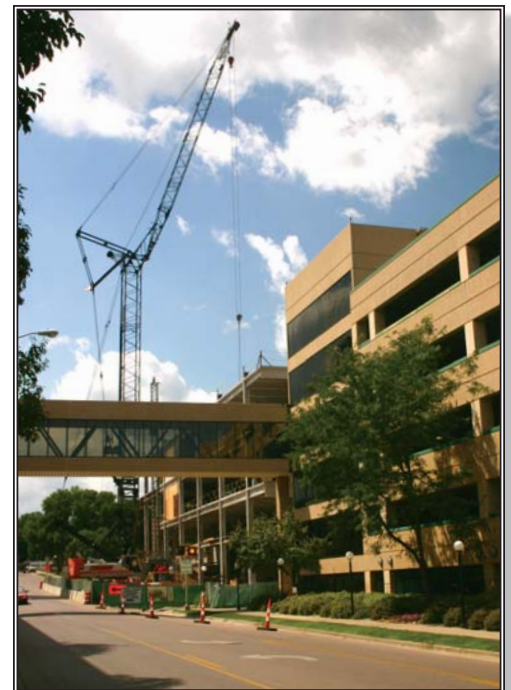
Healthcare construction includes the expansion of the Sioux Falls Surgical Center near the Avera McKennan campus.
