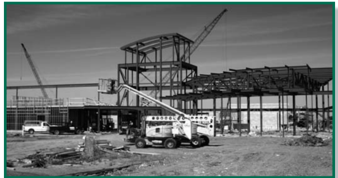
The new Harrisburg High School, scheduled to open in the fall of 2009, is currently under construction.
