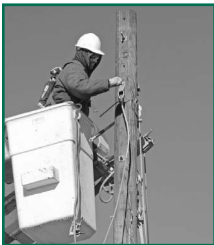
A Sioux Valley Energy lineman works in the cold at the top of a pole.
