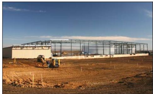
Variety Foods is constructing a distribution center in Sioux Empire Development Park VIII.
